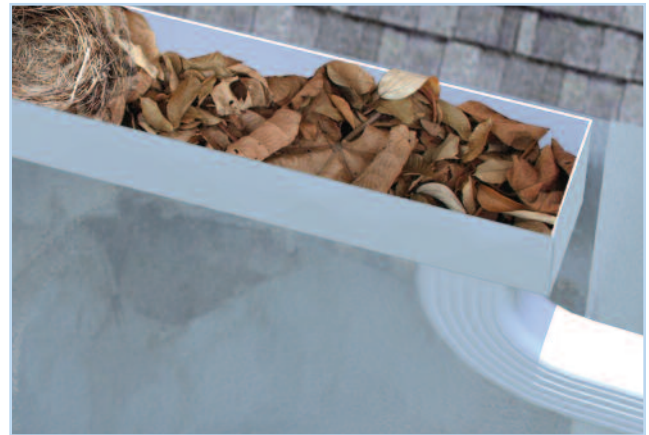
A clogged gutter can become a home for pests and prevents proper drainage away from the building.
