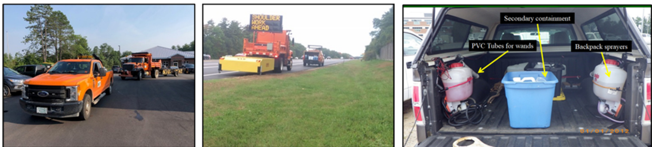
The photos on the left show the DOT support & safety vehicles provided to Mr. Cygan during herbicide activity. The photo to the right shows the application equipment used.
